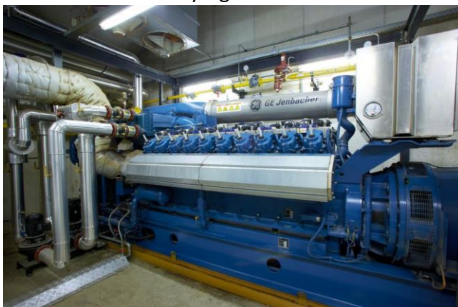
Figure 16 Cogeneration installation source: lekhabo.nl
